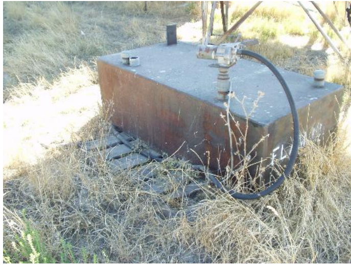
ABOVE GROUND FUEL TANK
