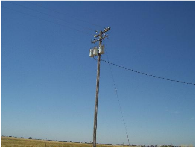
POLE MOUNTED TRANSFORMER NEXT TO SOUTHERN WELL VIEW TO NORTHWEST
