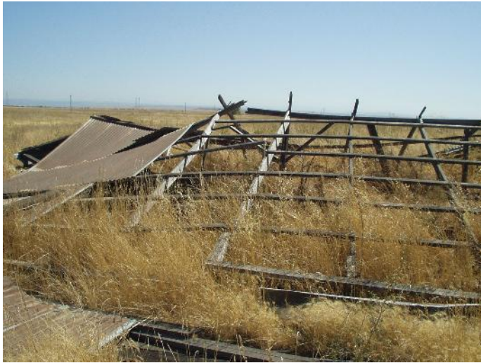
COLLAPSED STORAGE SHED IN WESTERN FIELD VIEW EAST
