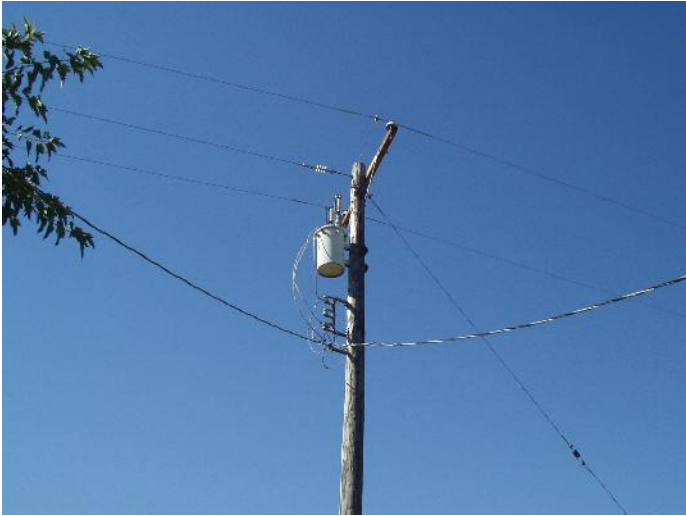
POLE MOUNTED TRANSFORMER ALONG HOUSE VIEW TO SOUTHEAST
