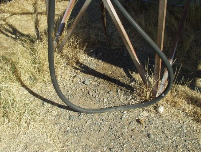
SMALL 1'X1' FUEL SOIL STAIN BENEATH ONE OF THE FUEL TANKS VIEW TO NORTH
