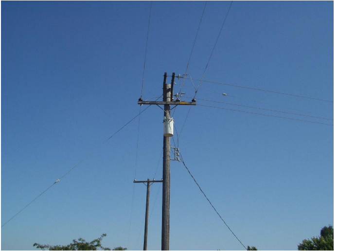
POLE MOUNTED TRANSFORMER ALONG THE NORTHERN BOUNDARY OF THE PROPERTY VIEW TO WEST
