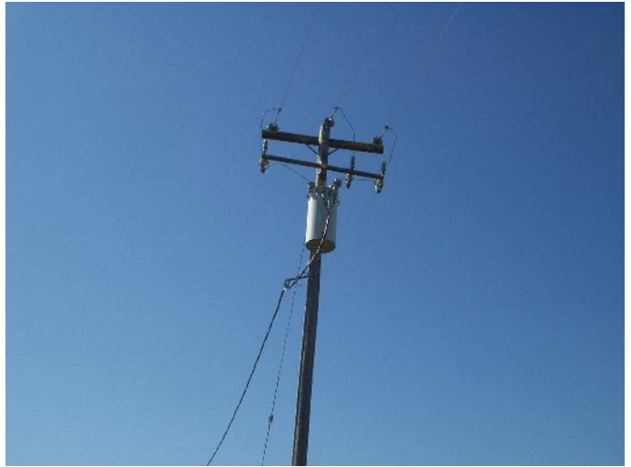
POLE MOUNTED TRANSFORMER ALONG NORTHERN WELL VIEW TO SOUTH
